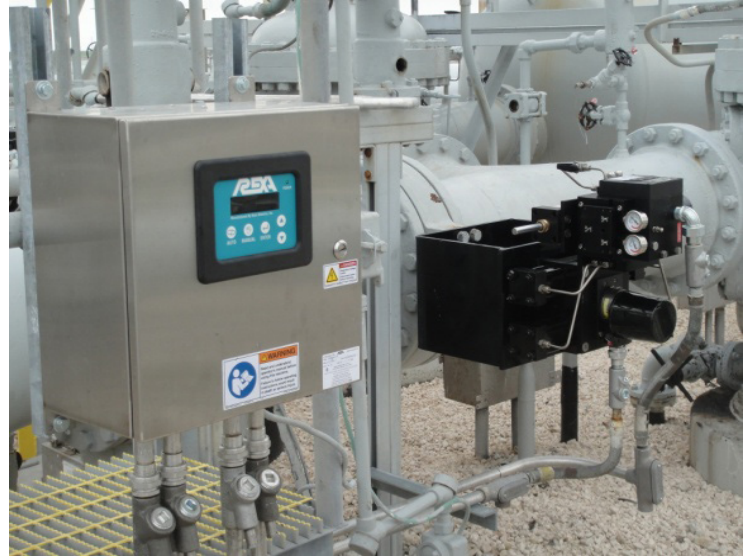
Field wiring is terminated inside the control enclosure
